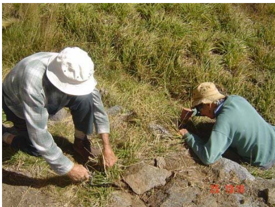
Carol Russell and Peter Melhuish clearing grass and weeds from around stones outside western door in preparation for re-grouting. This work was interrupted by rain and later, snow.
