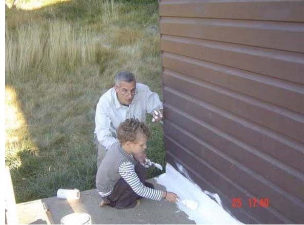
David Stuart and son, Albert, weatherproofing joint between patio slab and lodge wall.
